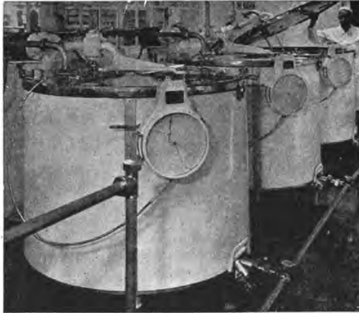
In modern dairies you find modern glass lined pasteurizers
