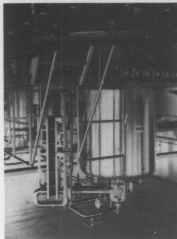
Schmidt-Bretten Food Deaeration System
