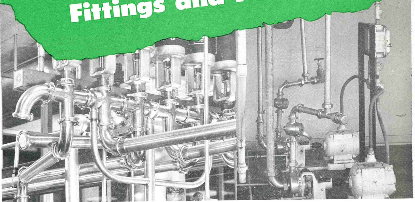
Battery of electrically-operated Tri-Clover compression valves with Tri-Clamp connections in a liquid conveying line.
