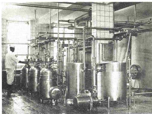
Figure 3. Processing facilities in Stainach milk plant.
