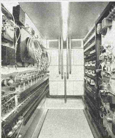
INTERIOR VIEW—CONTROL CUBICLE
